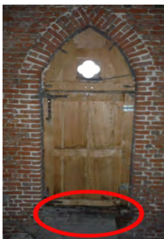
zolder [6]-west: lekken
