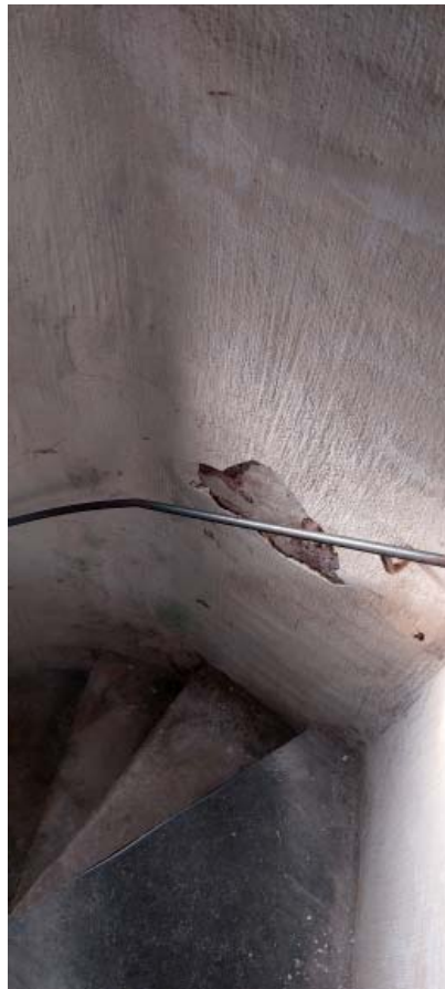
Fig. 55. Schade in draaitrap belfort, 2022 © ARTER
