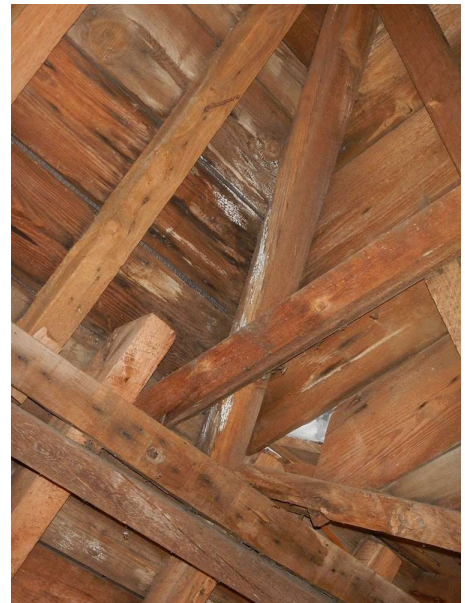
Beschimmelde beebording/hoekkeper dak [2]
