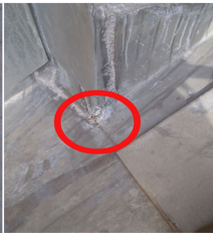
dak [3]-west monding zakgoot
