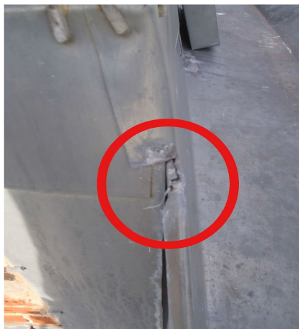
dak [3]-west monding zakgoot
