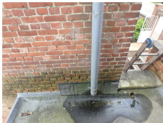
Dak [1]-noordwest: opspattend water.
