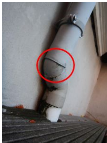
dak [1]-west: lekke afvoer
